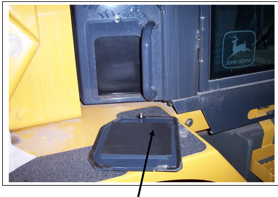
Outside air intake with louvers on door restricted by self adhesive foam panel
