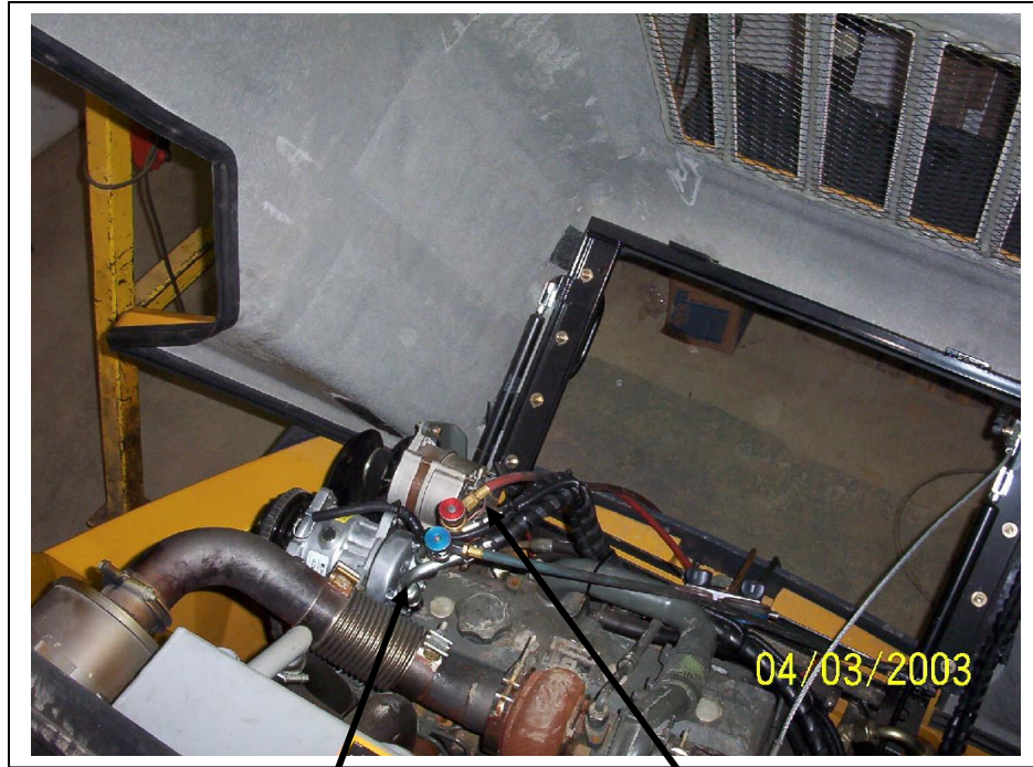
1/2" hose on compressor
